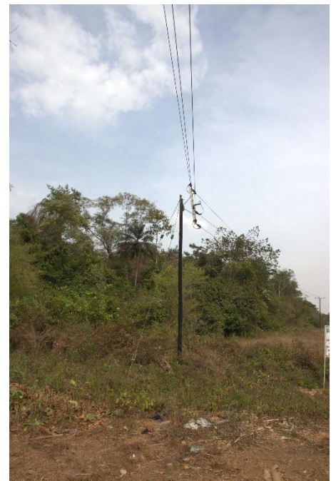
Damaged MV pole in Grand Cape Mount County
