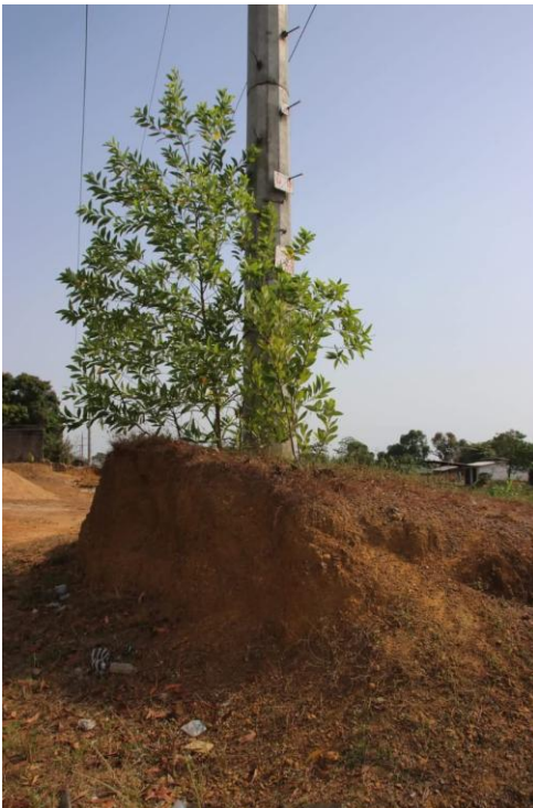
Dirt miners undermine a 66KV monopole
