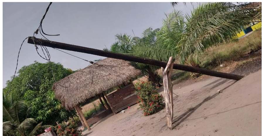
Damaged LV pole in Boimi Town, Robertsports Highway in Grand Cape Mount County
