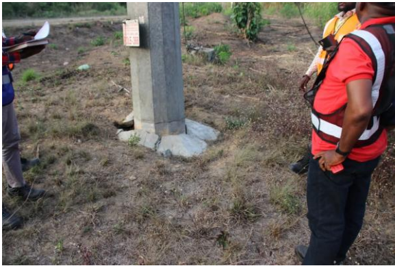
66KV monopole foundation failure
