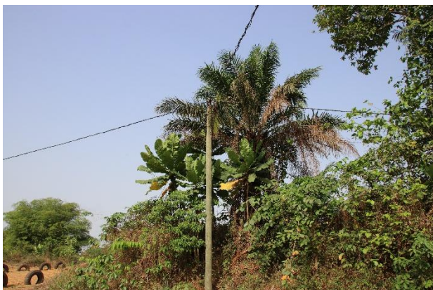
Vegetation interferes with LV line
