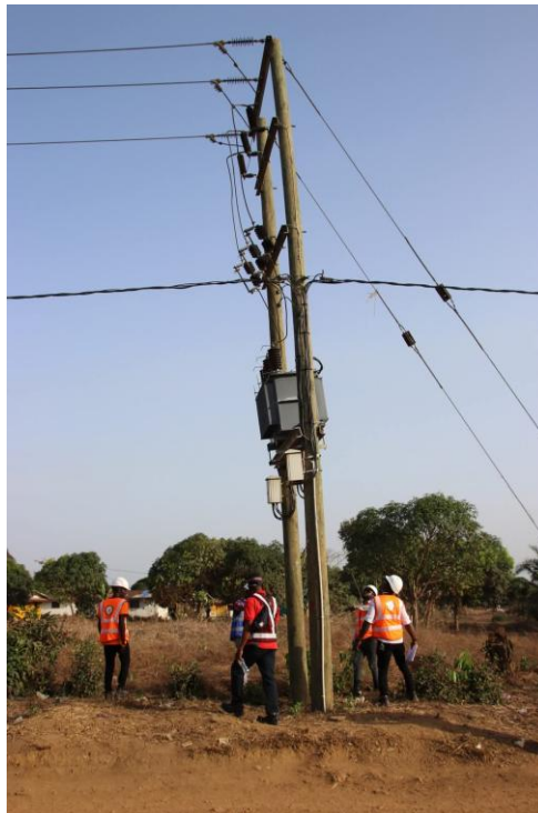
Leaning transformer poles
