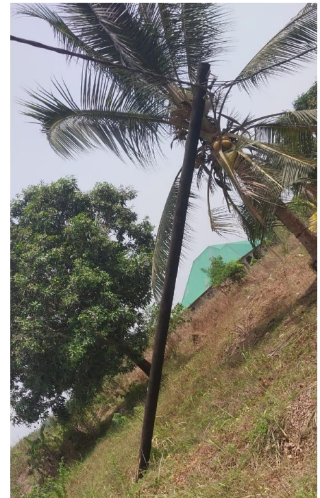
Leaning LV pole
