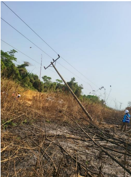
Damaged pole by bush fire
